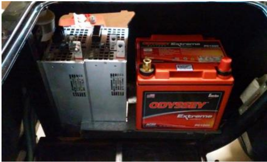
Figure 17. Photograph of the power supplies and battery mounted in the golf cart without golf cart batteries installed.
