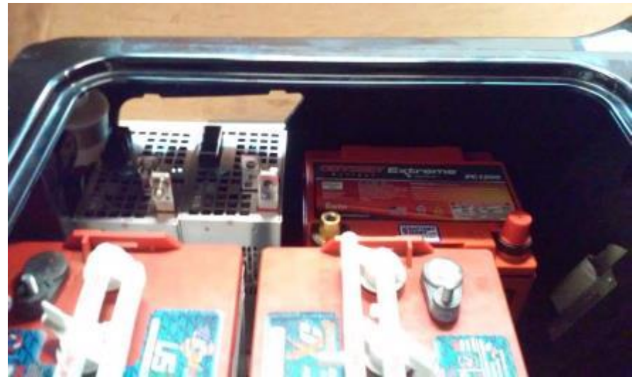
Figure 18. Photograph of the power supplies and generator battery mounted in golf cart with golf cart batteries installed.
